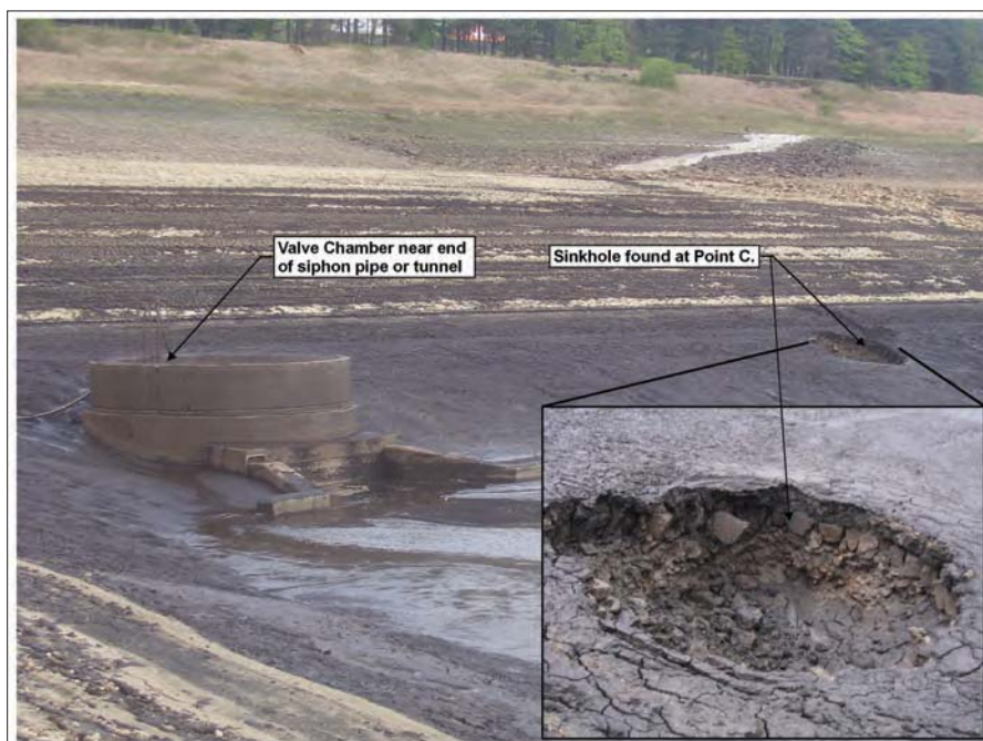
Figure 14. After the reservoir was drained, a sinkhole was found at Point C.
