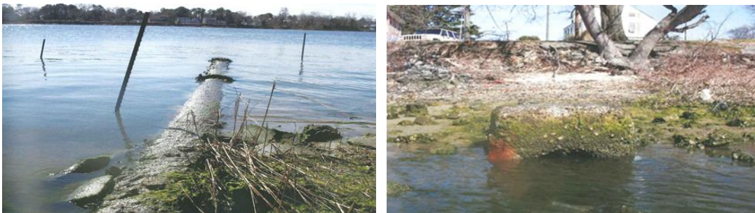
Storm Water Pipe Outfalls Submerged at Low Tide
