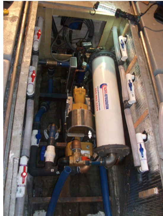
Figure 4: Pac-West unit in place with zone plumbing
