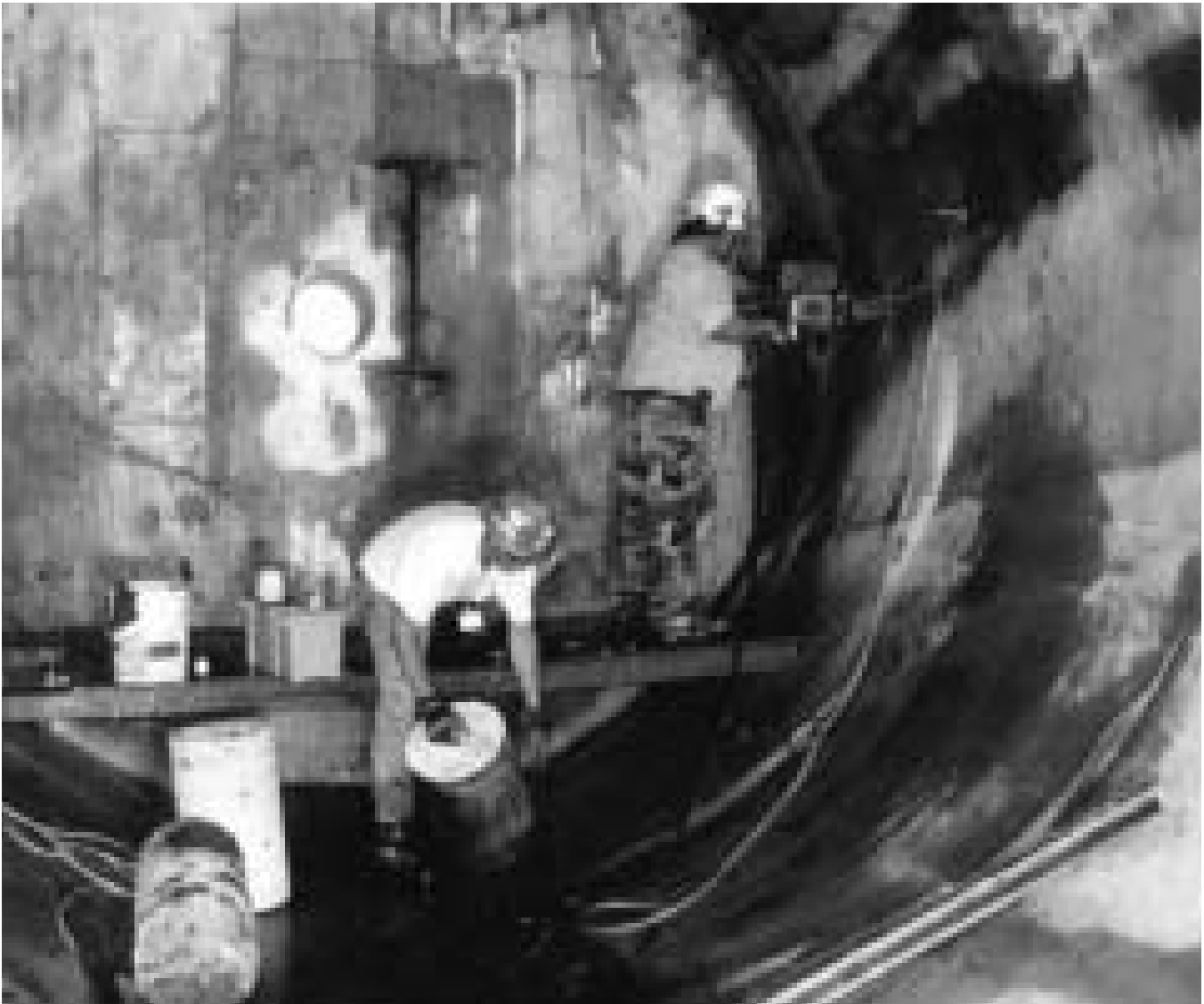
Operators cut the center pivot hole and two 4-inch-diameter wire access holes to allow set-up of the wire saw.
