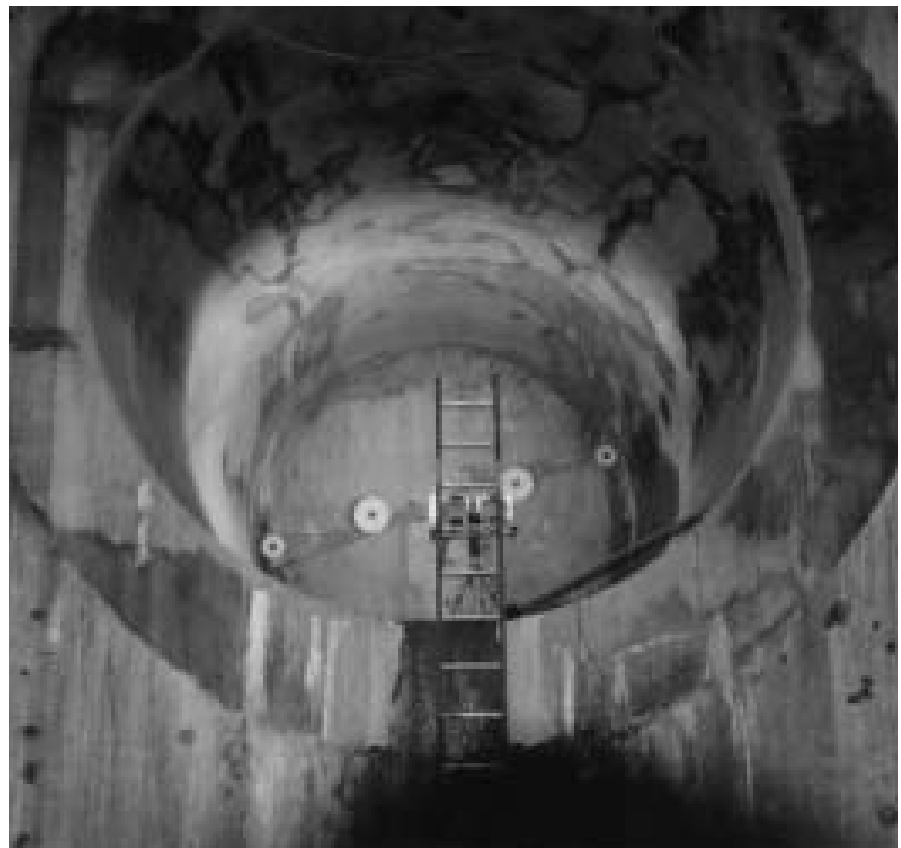
Top: Access to the new side of the tunnel was limited by an opening only 3 1/2 feet wide. Bottom: Wire saw set-up viewed from the new Shaft #6 side.
