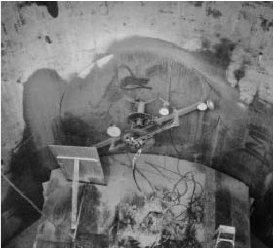
Top: Wire saw set-up viewed from existing Shaft #4. Bottom: Ninety percent of the cut is complete in the view from the existing shaft.
