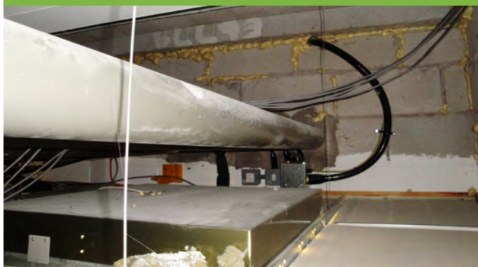
Foul water pipe in ceiling space above servers
