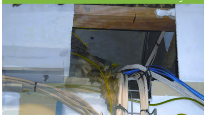
Holes into ceiling space in a server room; compromising fire suppression plus it will allow smoke into the server room if a fire broke out elsewhere in the building
