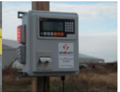
Step 9: Install controller and complete electrical connections. Apply power and weigh trucks
