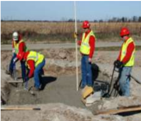
Step 4: Lay second layer of CA-6 stone, compact to 95%. Surface should be 11.5 inches below grade
