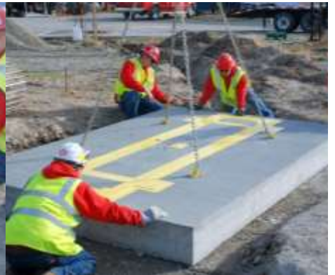
Step 6: Set the scale using 50' of masons twine to ensure it is parallel to the road
