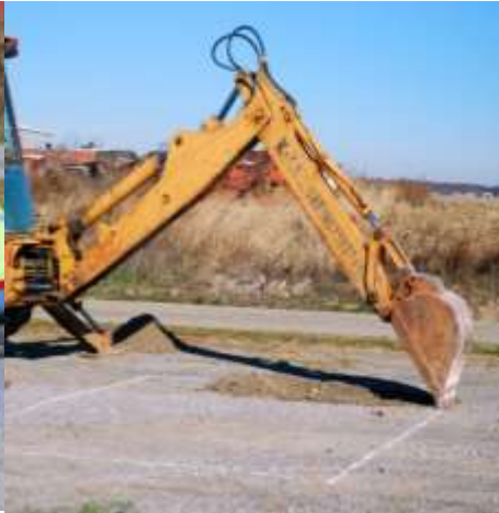
Step 2: Excavate and compact 14 X 10 foot hole 2 feet deep. Dig trench for home run cable and drains
