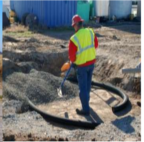
Step 3: Lay 4" drain tile and first 6 inch layer of CA-6 crusher run stone. Compact to 95%
