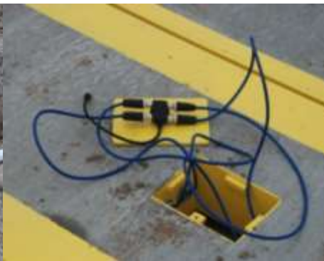
Step 8: Make watertight electrical connections at scale and controller. Back fill perimeter of scale, drains and conduit runs
