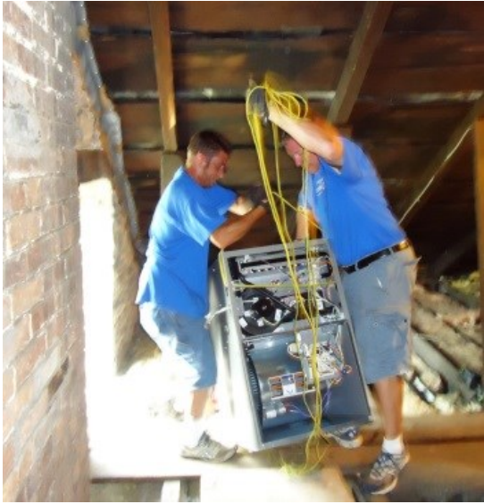
Getting the new furnace through the small opening to the Stone Academy attic was no easy matter. For more information see page 2.
