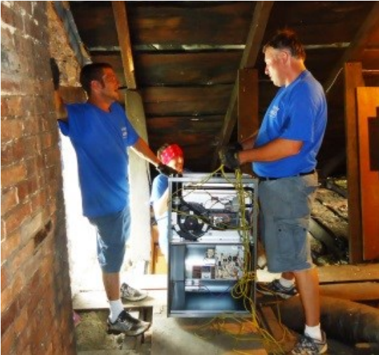
Interesting juxtaposition of new heating technology with 200 year old roof rafters and sheeting.
