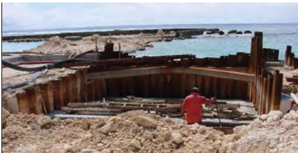
Mainstreaming climate change considerations into infrastructure design will help to minimise funding costly repairs if damages occur from extreme weather events
