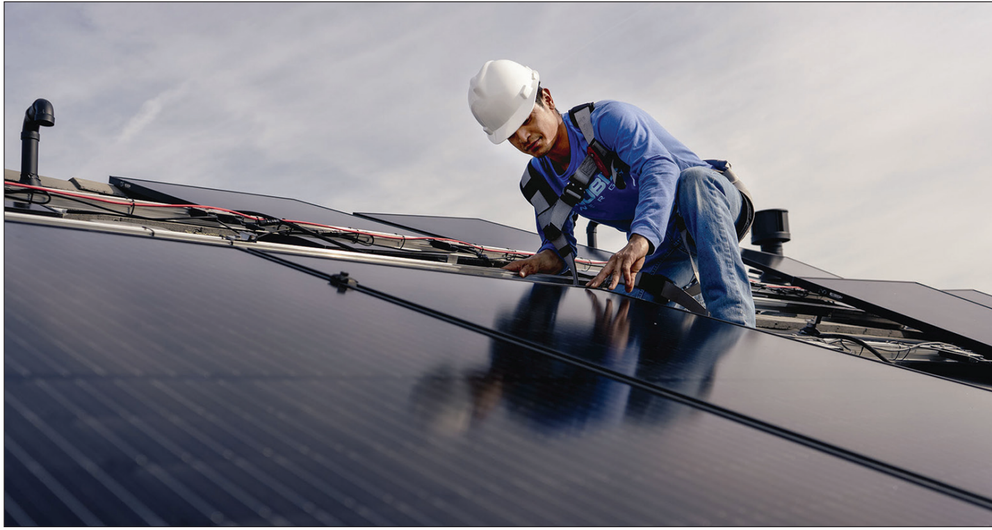
PHOTO COURTESY OF KUUBIX ENERGY, INC.
