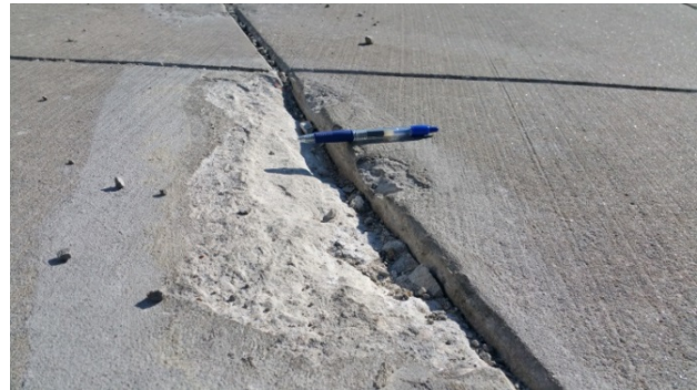
Figure C-9: Edge Spalling Immediately Inside Gate D
