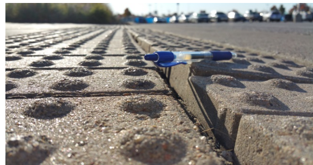
Figure C-3: Uneven Paver Settlement at Pedestrian Traffic Way
