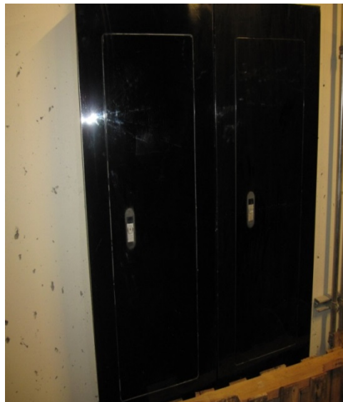
Figure E-8: Existing Unlabeled Panelboard
