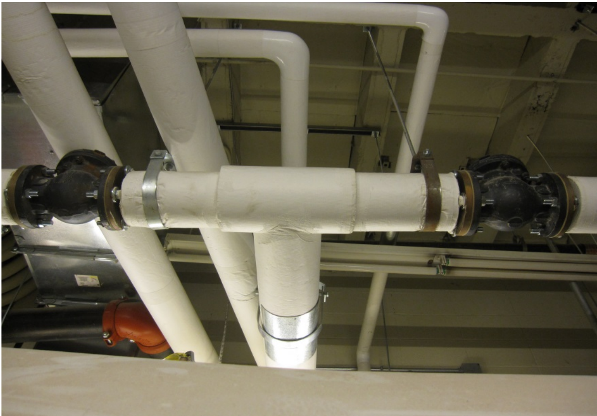
Figure M-1: Piping Hangers Missing Insulation Shields
