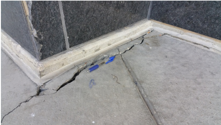
Figure C-5: Joint Spalling Along North Building Facade
