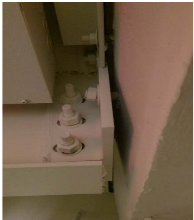
Figure S-4: Concrete Anchor Pulling Out of Concrete Beam
