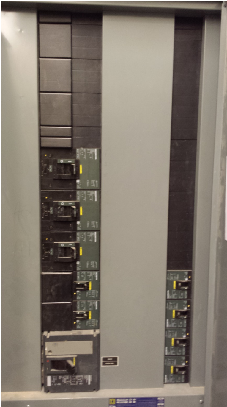
Figure E-9: Unlabeled Breakers in Distribution Board B1C3A
