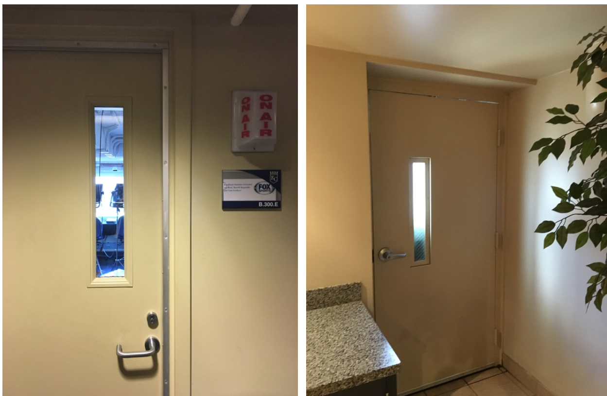
Figure AI-10: Typical Hollow Metal Door Conditions
