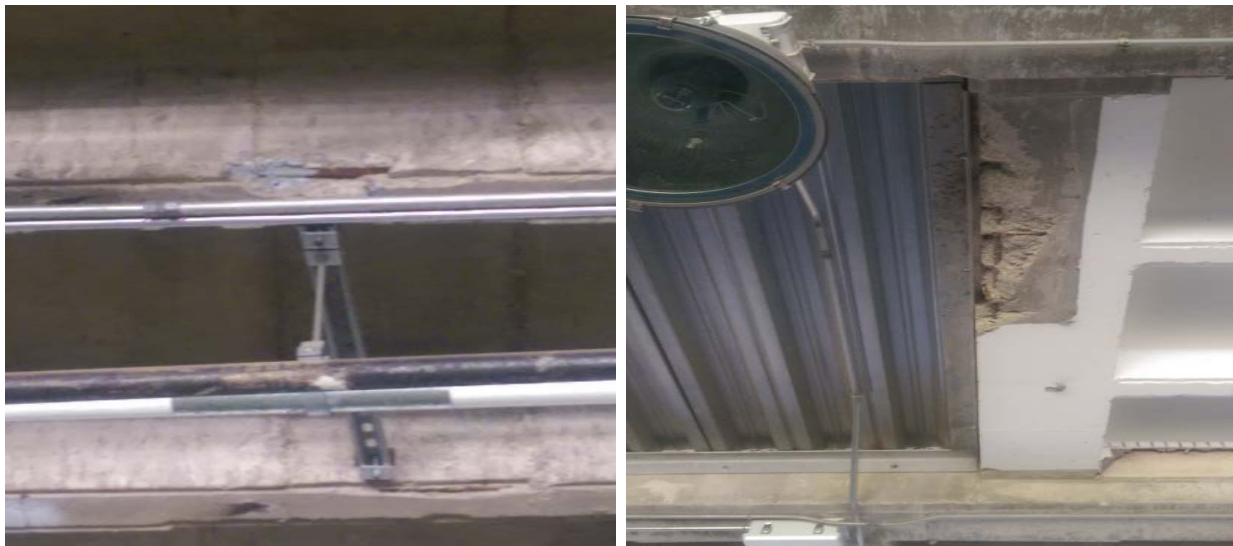
Figure S-2: Concrete Spalling, Exposing Reinforcement
