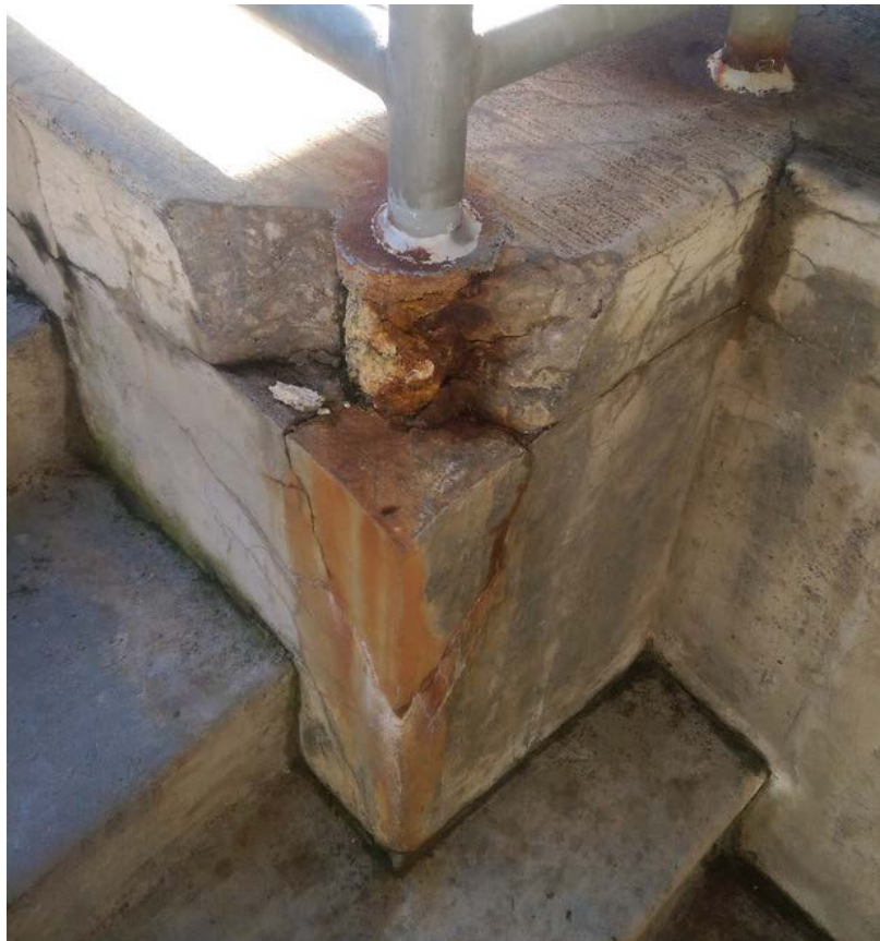
Figure S-5: Corrosion and Concrete Spalling of Guardrail
