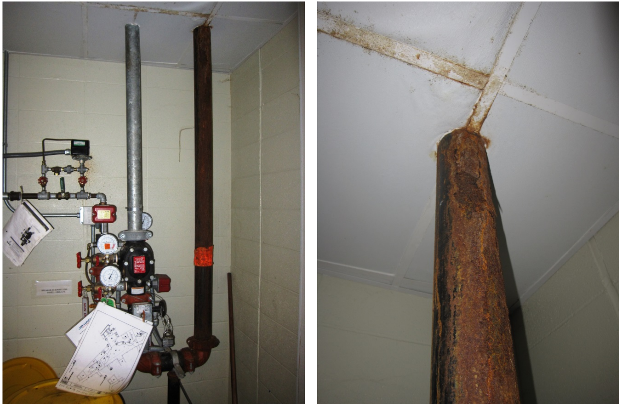
Figure M-6: Dry-Pipe Sprinkler Valve System and Corrosion of Steel Piping
