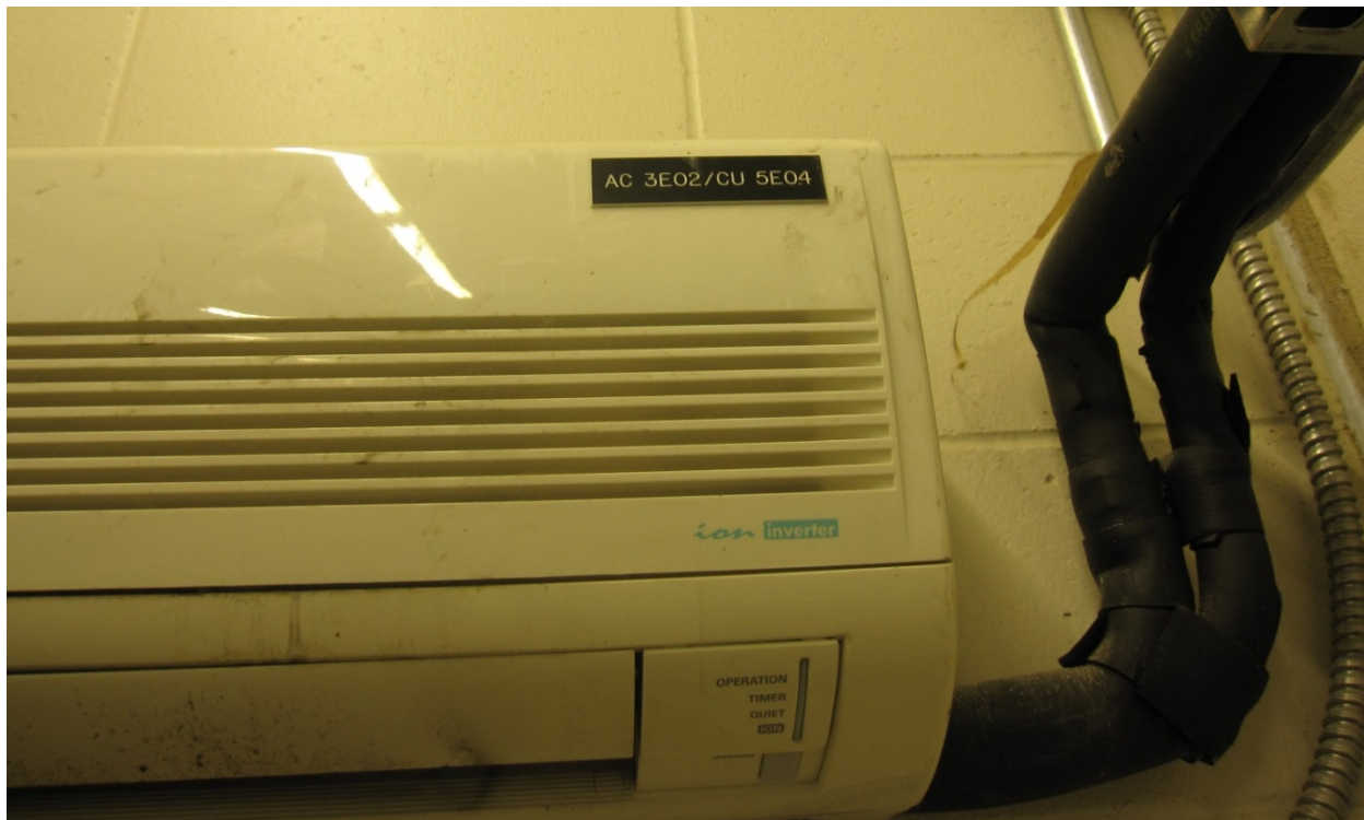
Figure M-7: Wall Unit AC 3E02
