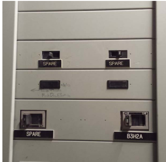
Figure E-7: Switchboard B3M with Blank Covers Not Identified as Specs
