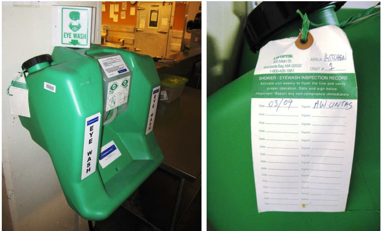
Figure M-5: Wall-Mounted Eyewash Station and Verification Tag
