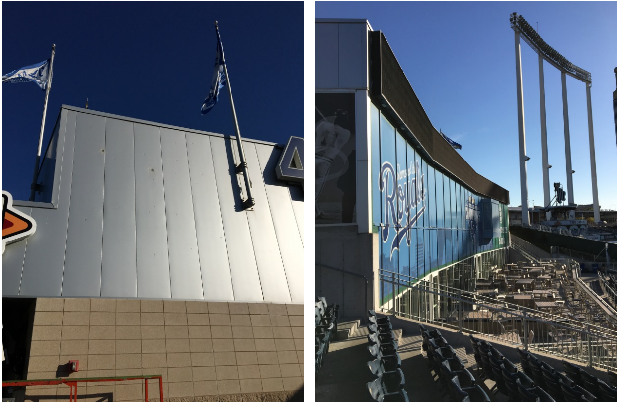
Figure AF-5: Metal Panel and Storefront System at Hall of Fame Structure
