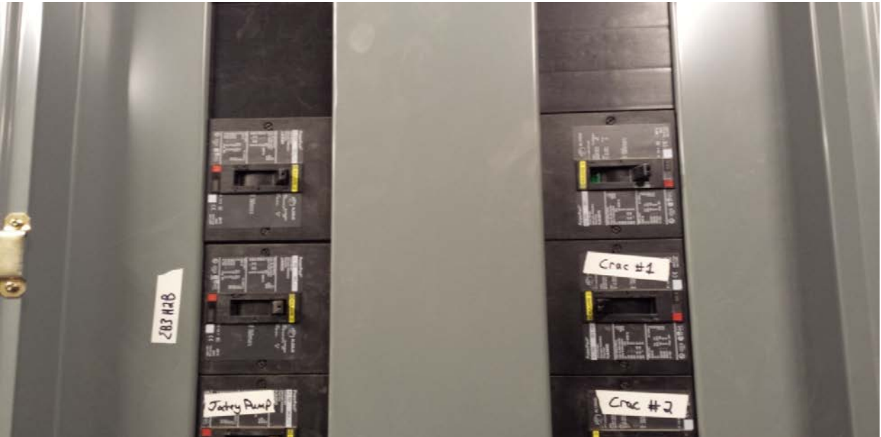
Figure E-3: Distribution Board EB3H2B
