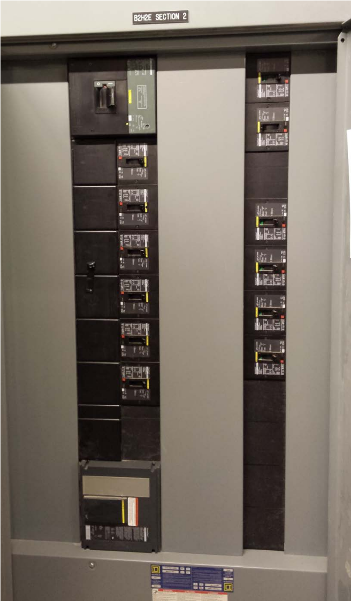
Figure E-5: Distribution Board B2H2E Section 2 with Unlabeled Breakers
