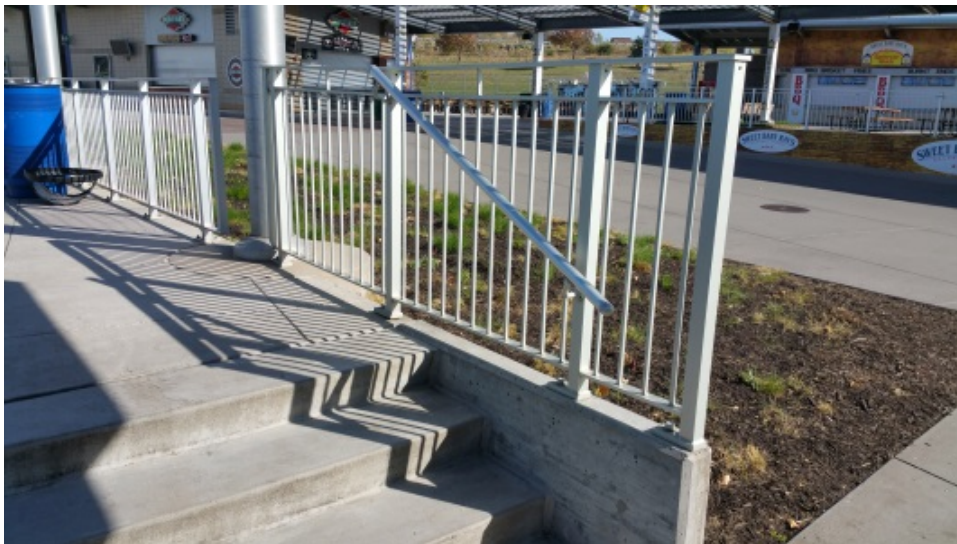
Figure L-3: Unsecure Hand Rail at Stairs
