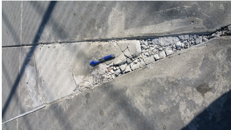
Figure C-6: Damaged Pavement Patch Outside of Gate D
