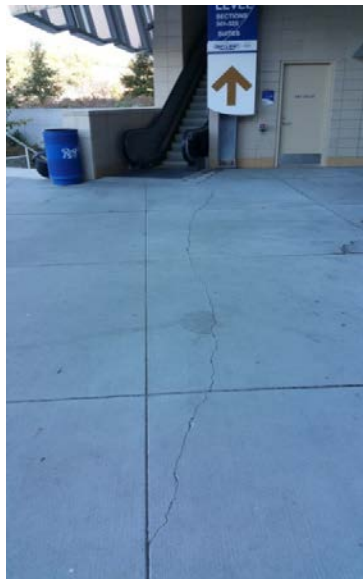
Figure C-7: Crack Near Spiral Ramp Behind Gate 3
