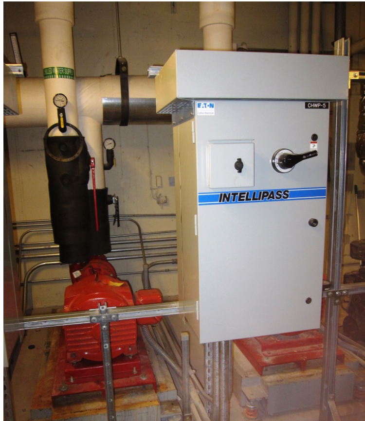
Figure M-2: Chilled Water Pump, CHWP-5
