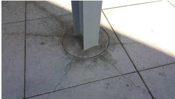
Figure C-8: Cracking Radiating Out From Column Foundation
