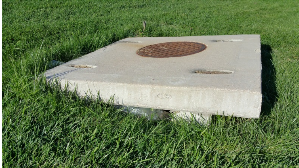
Figure L-4: Dislodged Storm Structure
