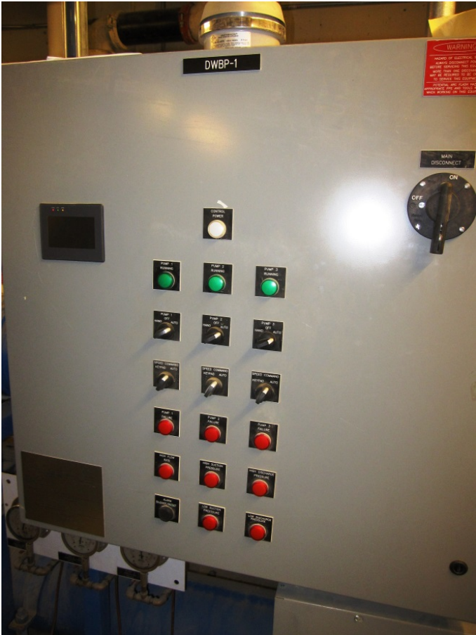
Figure M-3: Domestic Water Control Panel
