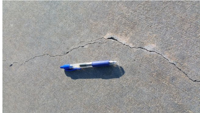
Figure C-1: Minor Cracking at Concrete Walkways
