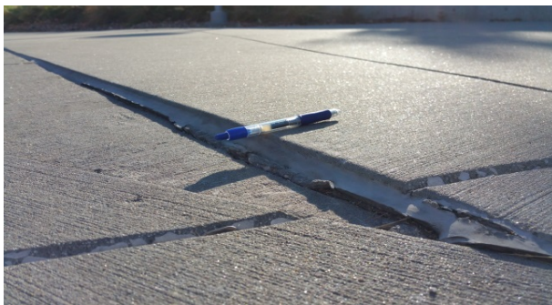
Figure C-2: Joint Fault at Pedestrian Traffic Way
