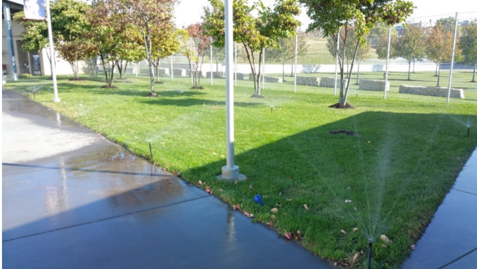
Figure L-2: Irrigation System in Operation
