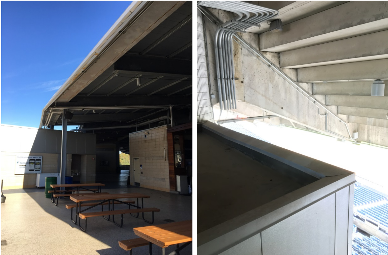
Figure AR-2: Roof Coping and Fascia Panels at Roof Eaves and Parapets
