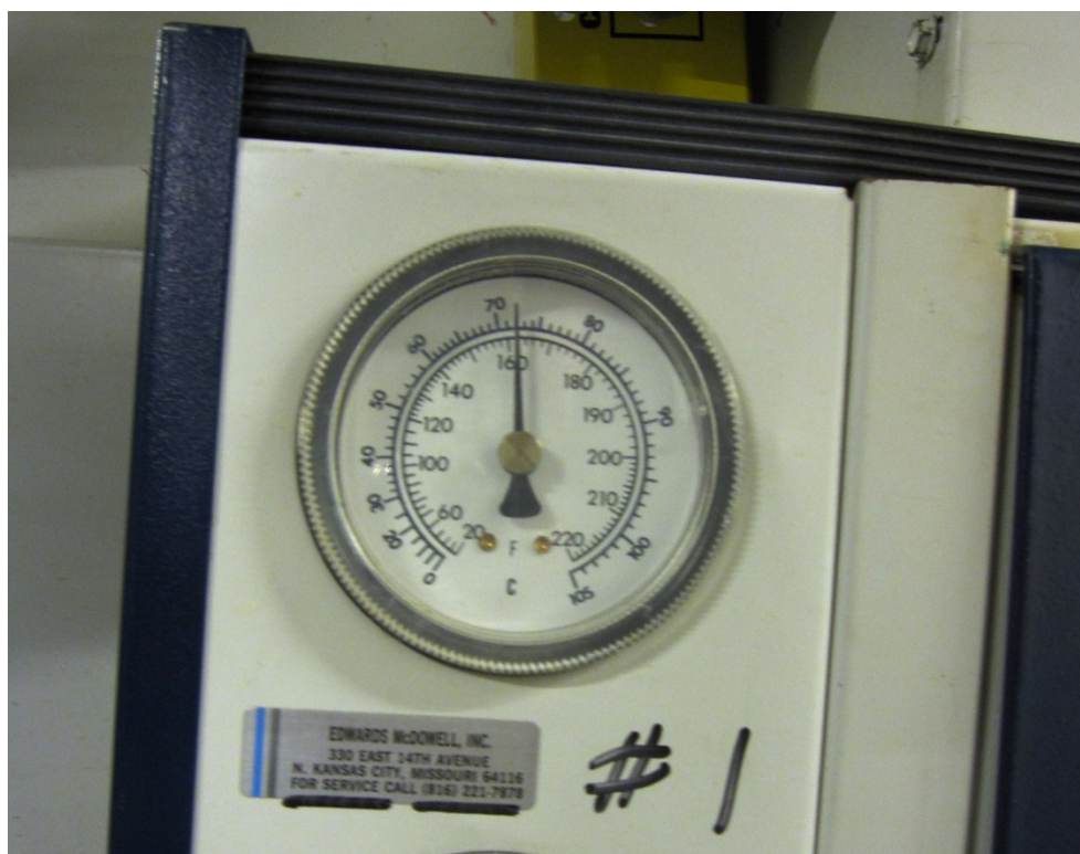
Figure M-4: Hot Water Boiler Temperature Gauge
