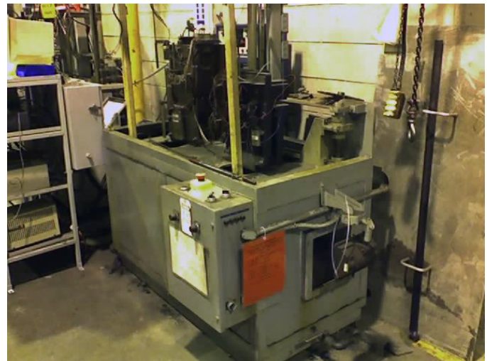
Figure 3. 200 Gallon Tank Filled with Envirotemp FR3 fluid
