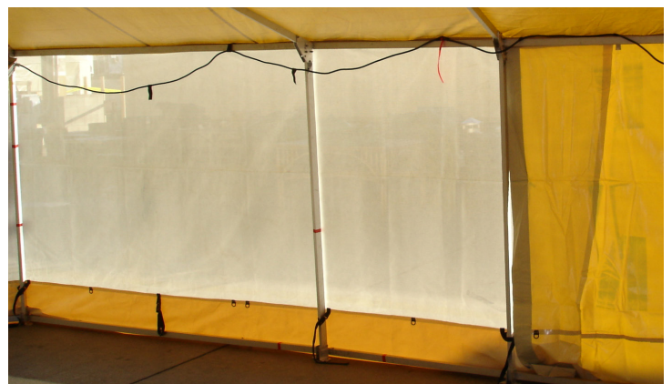
CL-SW H1935 installed in shelter
