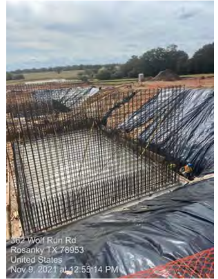
WTP/RWI - Flow Equalization Basin
