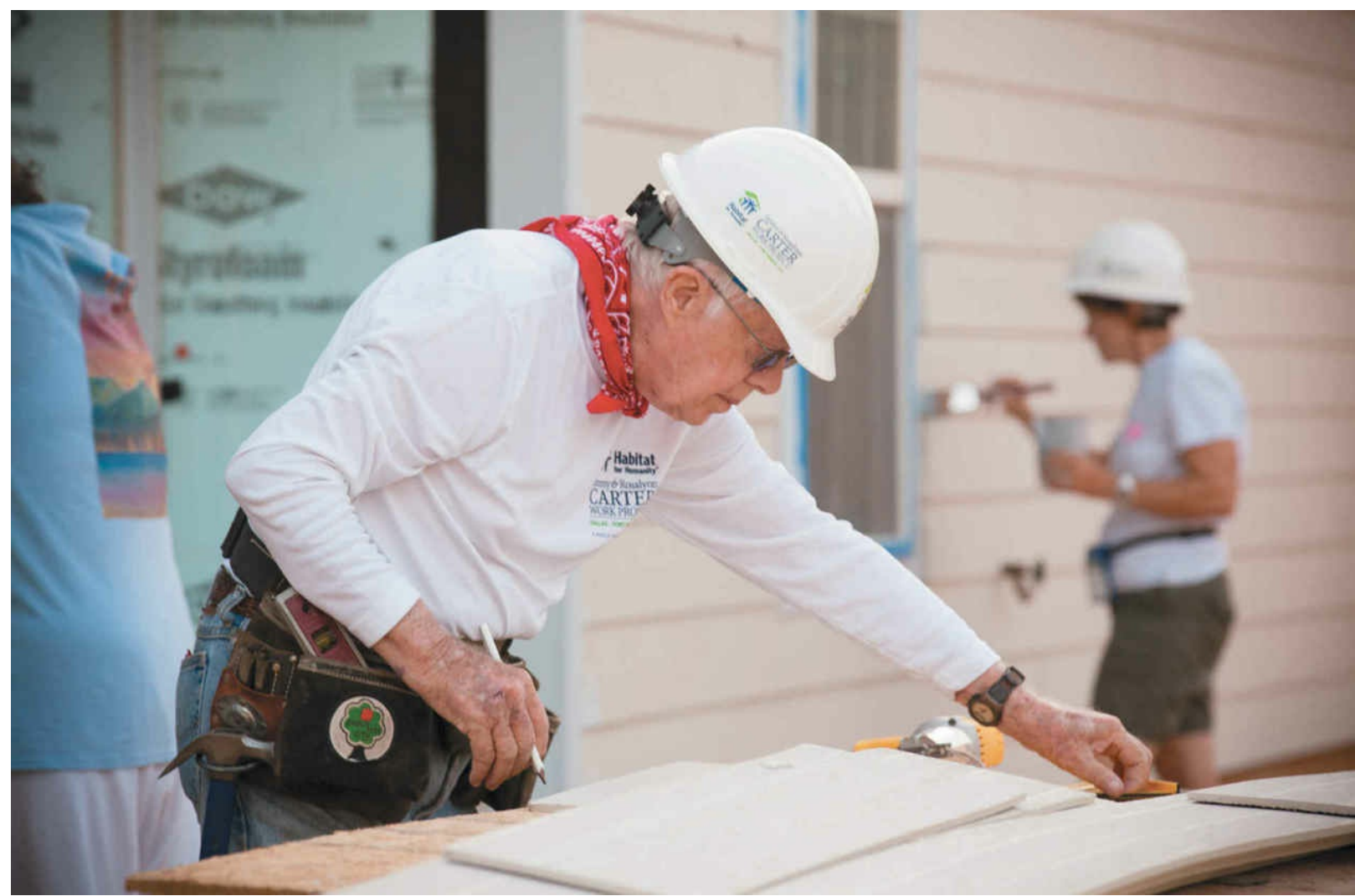
Installing siding on a new home during the 2014 Jimmy & Rosalynn Carter Work Project.
