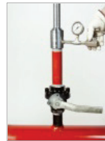
Figure 4.54. Installed Bleeder Valve
