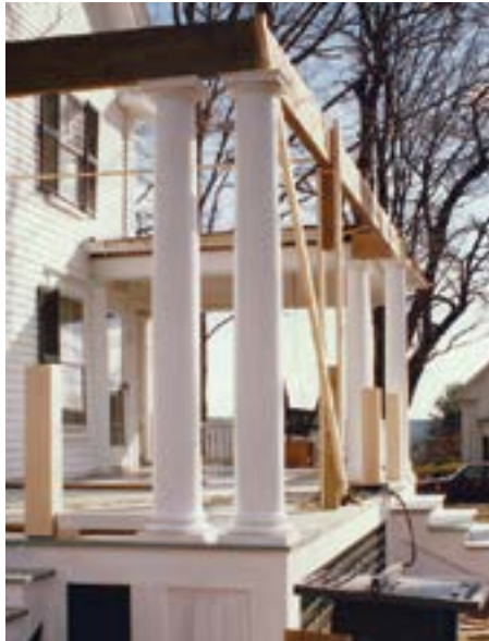
Installing columns at a job site. The blanks are turned from hollow tubes that are coopered from 10 individual staves
