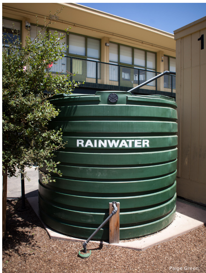
Rainwater cisterns at a schoolyard in San Francisco, California provide water for irrigation and opportunity for students to learn about water conservation.
