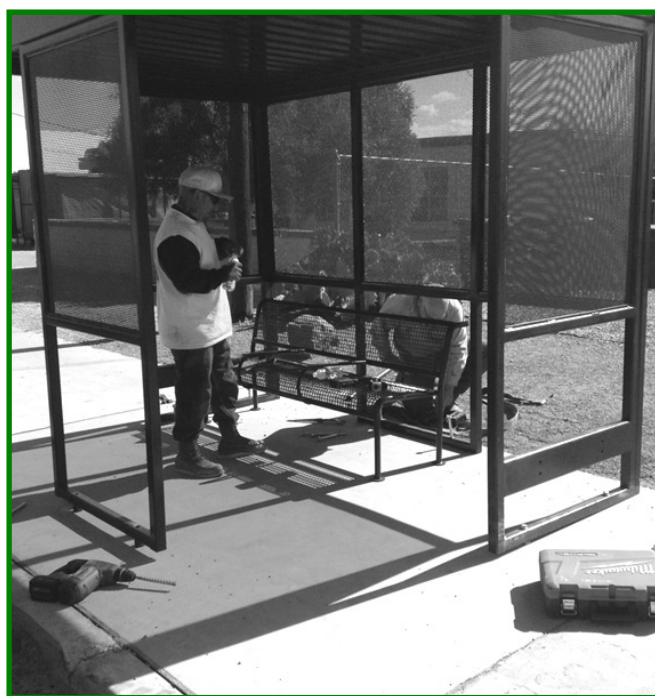
Thanks to the organizing work of student leaders at the El Rio Learning Center in Tucson, AZ, the city added this bus shelter to the bus stop across the street from their school. They are still fighting for a bus schedule that better meets students' needs.
