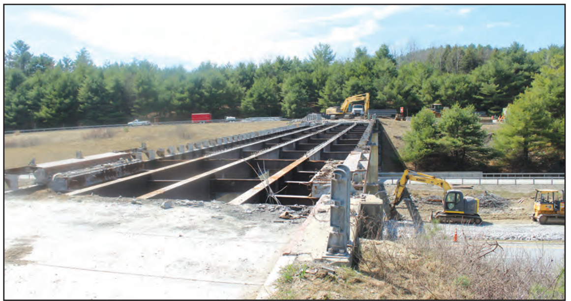
The reconstruction of the bridge crossing the Adirondack Northway at Riverbank will keep the southbound ramp at Exit 24 closed through November. Mirror staff photo.
