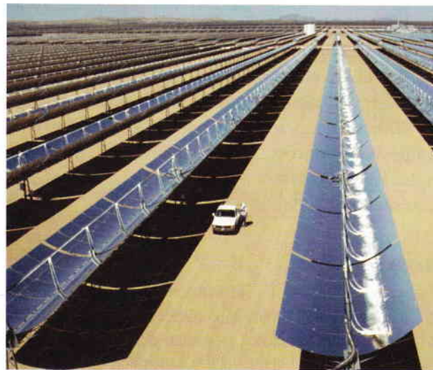
Solar energy power plant in California
