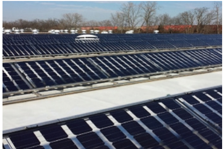
Figure 7. Bifacial PV on white reflective rooftop Source: Prism Solar 5th PVPVC Santa Clara CA 2016
