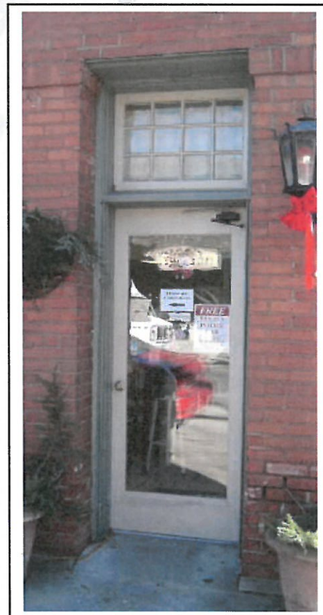
Right: Details such as transom windows allow for additional interior light and help to add character to an entrance. These features should be maintained and preserved.
