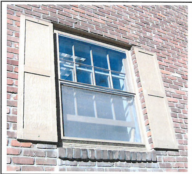
If shutters are used, they should be large enough to cover the window if closed.
