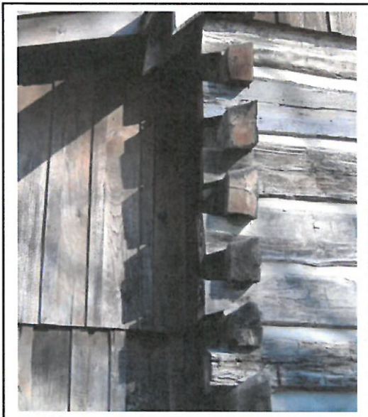
Some materials in Nashville, including log and some vertical batten siding, were traditionally left unpainted.
