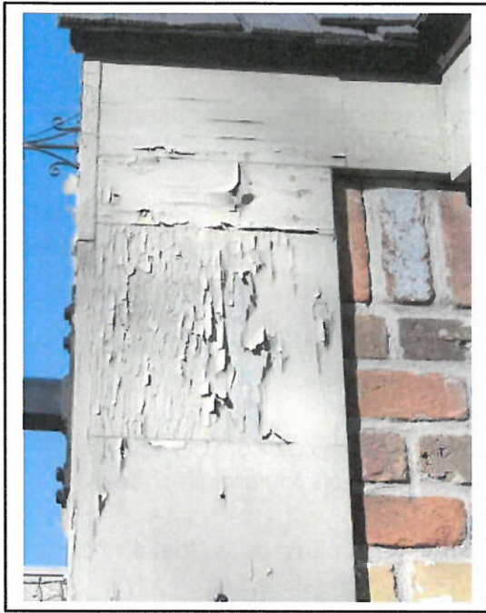
This cracked, alligatored paint is nearing the end of its life span.
