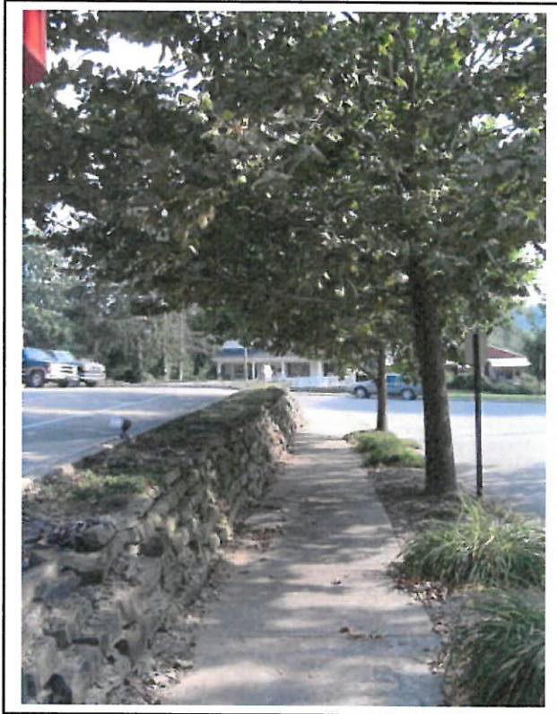
This stone retaining wall separates pedestrians from parking, but also serves as a barrier. Steps between the two levels would improve pedestrian access.
