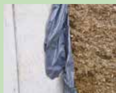
Lining the clamp walls with side sheets before filling the clamp is a key step to reducing air ingress.
