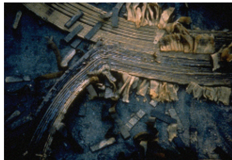
Figure 2-3. GIC Damage to Transformer During 1989 Geomagnetic Storm
