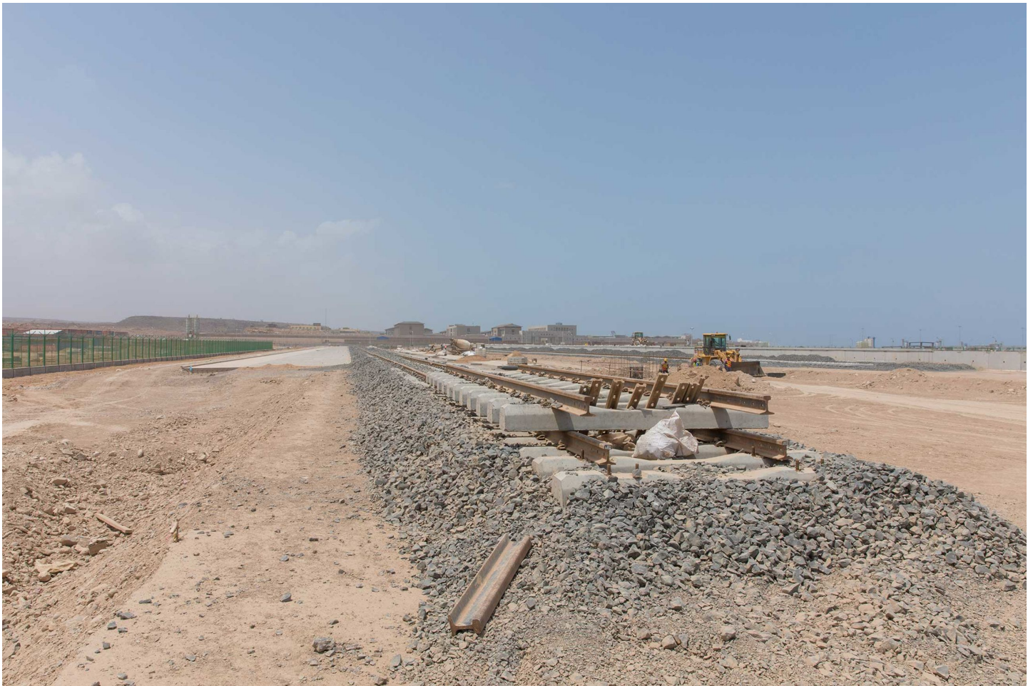
An unfinished rail line near the Chinese People's Liberation Army support base. Photographer: Sarah Waiswa for Bloomberg Markets
