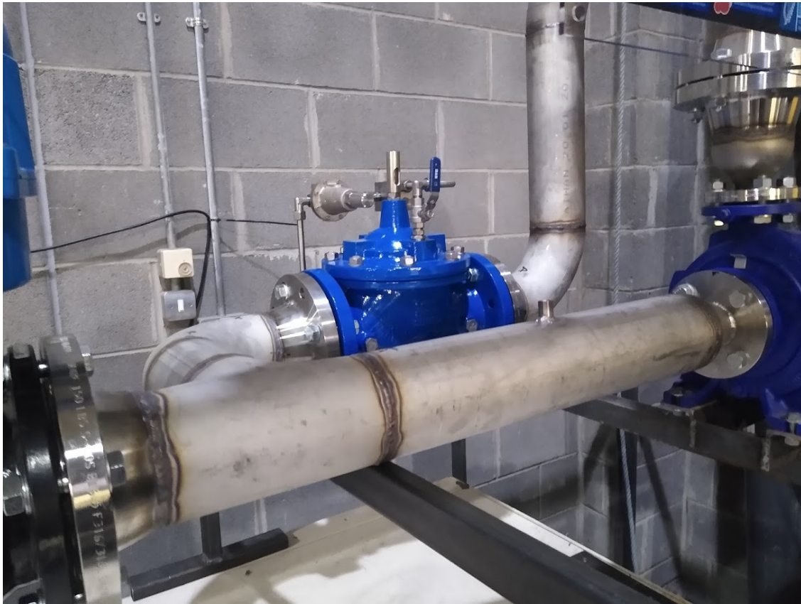
Upgraded test rig with PAT in parallel to PRV
