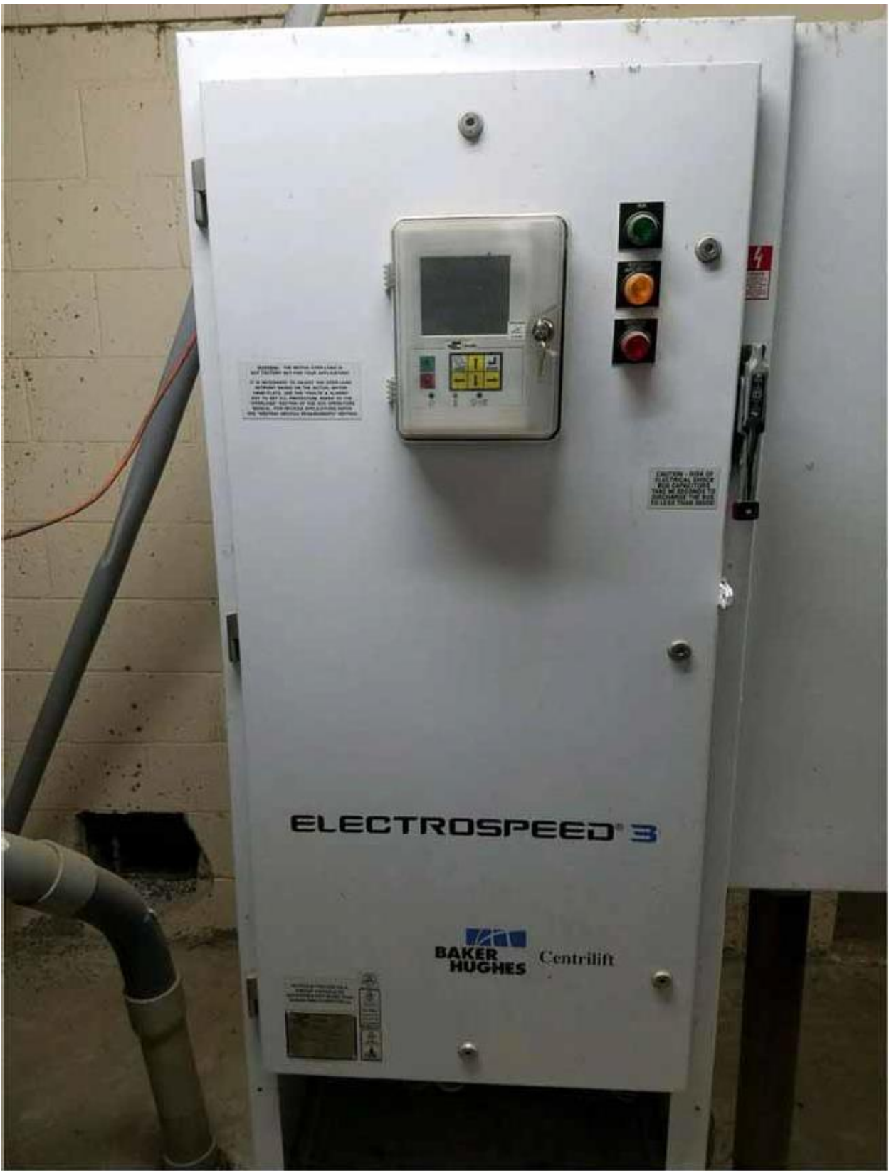
Images of existing variable frequency drive controller (VFD) inside well house.
