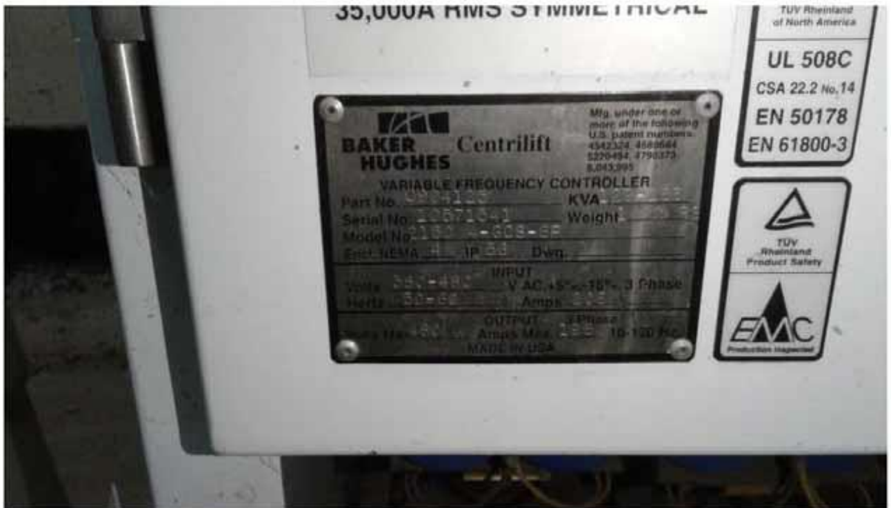
Images of existing variable frequency drive controller (VFD) inside well house.
