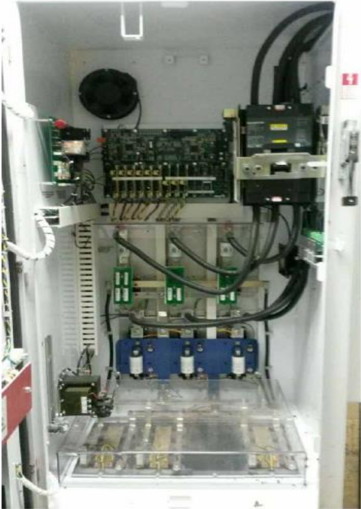
Images of existing variable frequency drive controller (VFD) inside well house.
