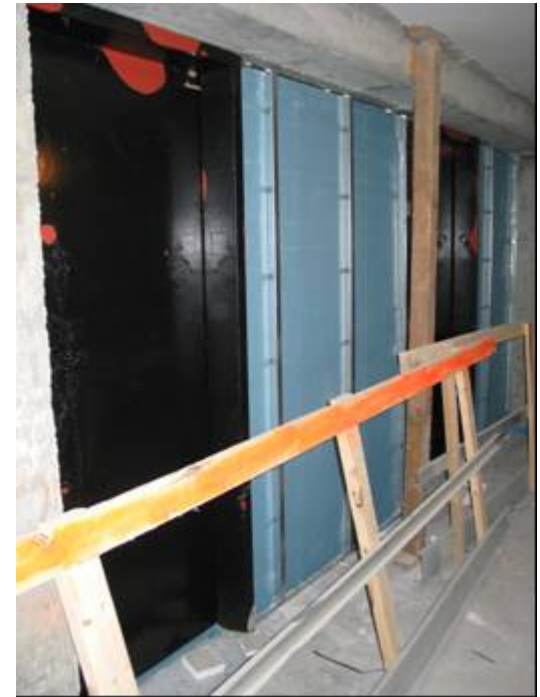
...to entrances installed and the shaft enclosed, without a platform
