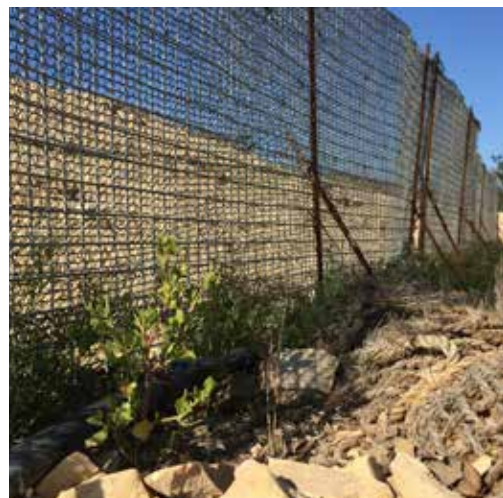
Coyote bush ( Baccharus pilularis ) is planted between fog drip netting and erosion control waddles. Coyote bush is a hardy and resilient plant making it an excellent candidate for early restoration succession.
