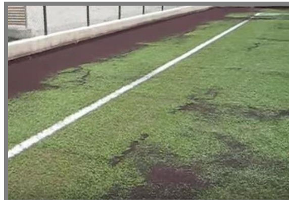
“Second field synthetic turf field, no longer playable, requires complete refurbishing after same rain storm ”
