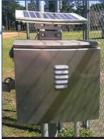
Pictured above is one of the Lone Star Groundwater Conservation District's Periodically Accessible Monitors (PAMs). The District has a total of eight PAM units located throughout Montgomery County, which enables the collection of land subsidence data.
