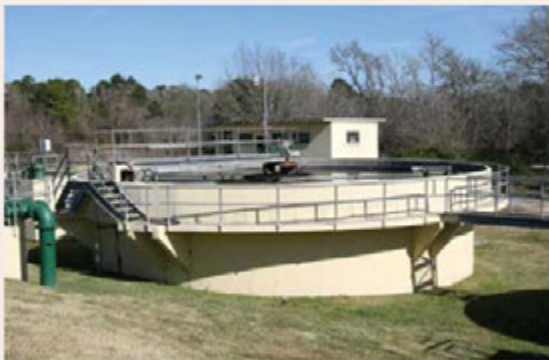
Photo 3: Next, the effluent flows into the contact chamber. It is at this stage that chlorine is injected to kill any bacteria.
