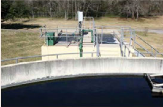
Photo 2: Once primary treatment is complete – water enters secondary treatment at the final clarifier.
