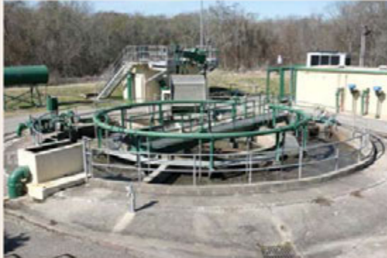
Photo 1: Treatment Plant #1. First stage of wastewater processing. Raw sewage enters plant and aeration chambers.
