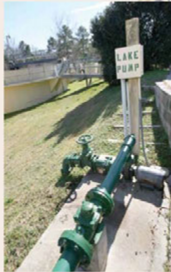
Photo 4: Effluent pumps deliver water from the contact chamber to the holding pond.
