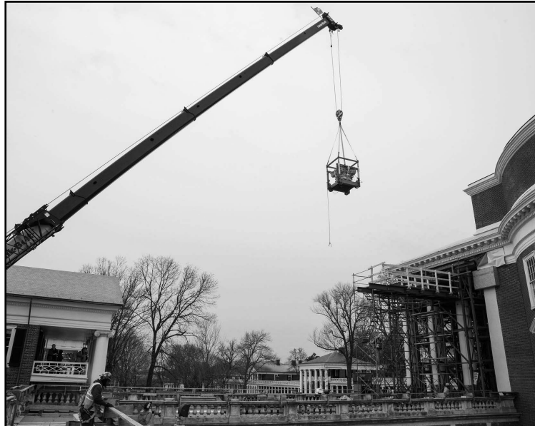
Pictured: Loathsome construction (destruction?) takes its toll on the surrounding areas under the guise of 'beautification'. Photo Courtesy of pages.shanti.virginia.edu
