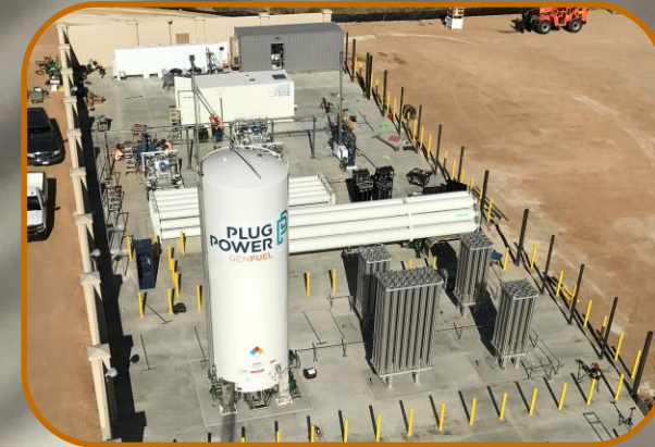
Skid: Modular Hydrogen System
