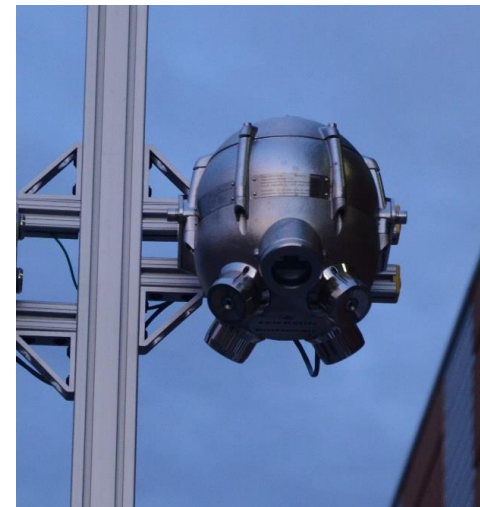
Commercial ultrasonic leak detector installed at NREL
