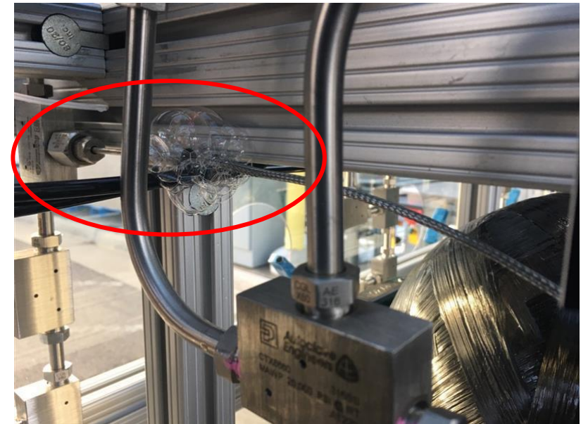
Small leak identified by a soap solution
