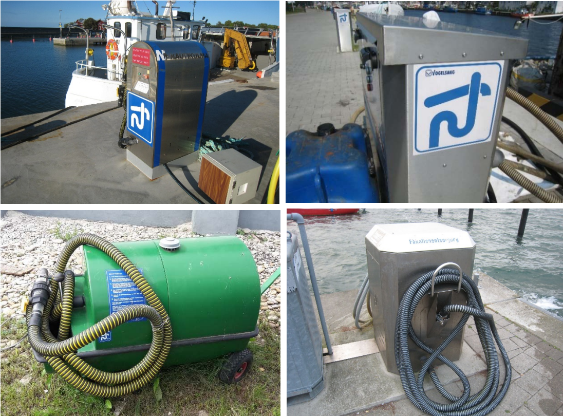
Different pump-out solutions for the reception of sewage at the harbours of Byxelkrok, Darlowo, Kappeln and Toila.
