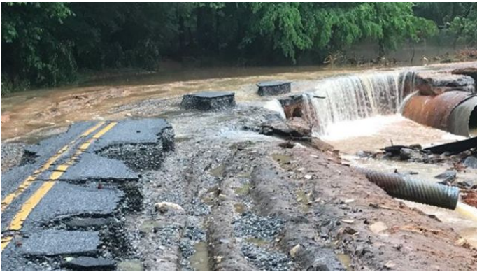
Photos, video | Flooding and flood damage in WNC (/news/local/gallery/photos-video-weekend-flooding-in-wnc)
