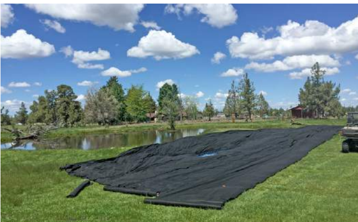
Installation of landscaping cloth to cover the entire bottom of a Redmond area irrigation pond in an attempt to solarize yellow floating heart.
