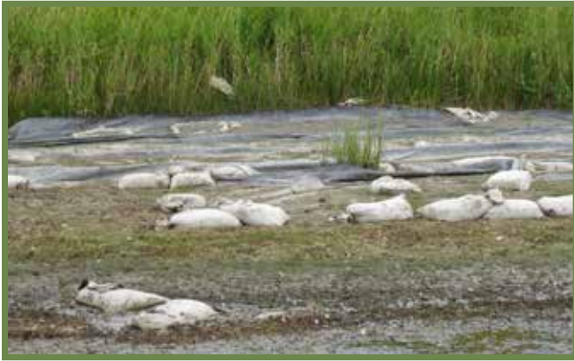
Figure 22a. Benthic barrier held down by sandbags (Photo credit: US Army Corp of Engineers).
