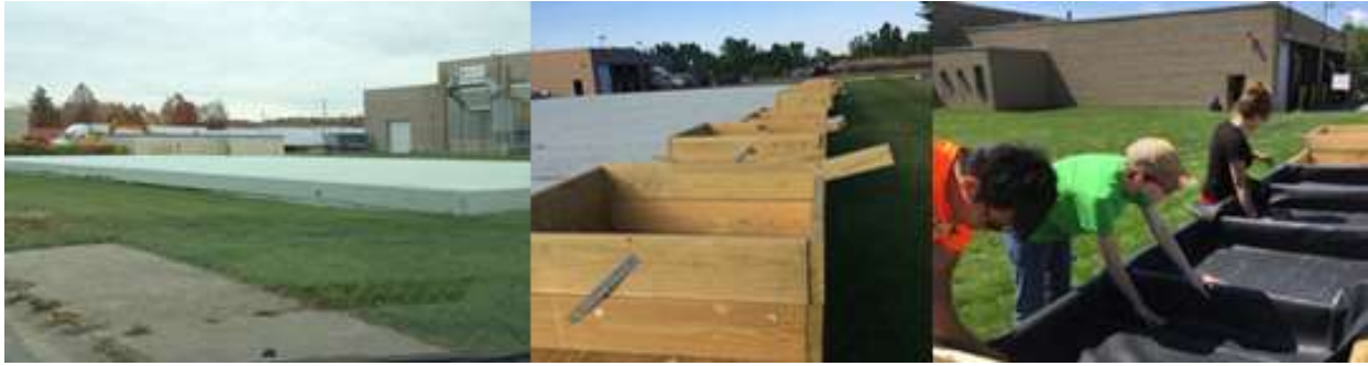
Figure 1. From left to right: Test site before construction, framework, and waterproofing membrane.
