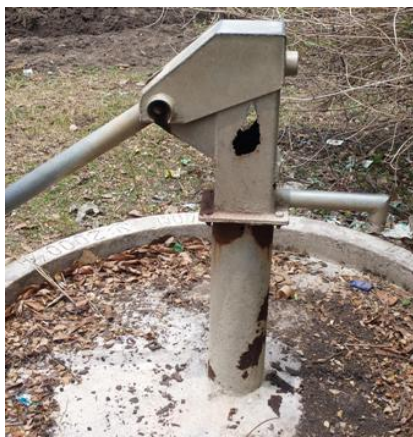
Pump well broken
