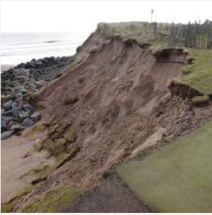
Erosion at Montrose
