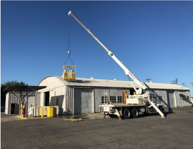
Lindsay maintenance staff initiated pressure washing and painting of the Lindsay yard buildings
