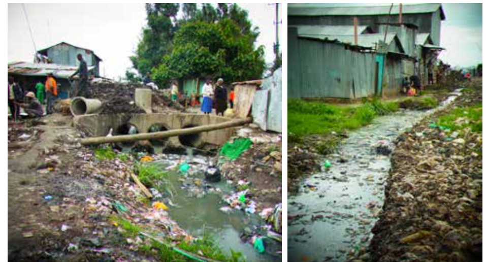
Figure 26(left): stream and open sewage in its way between Milimani and Zone 48. Figure 27(right) open drainage collapsed. ©Z.G.Blanco, CURI 2012
