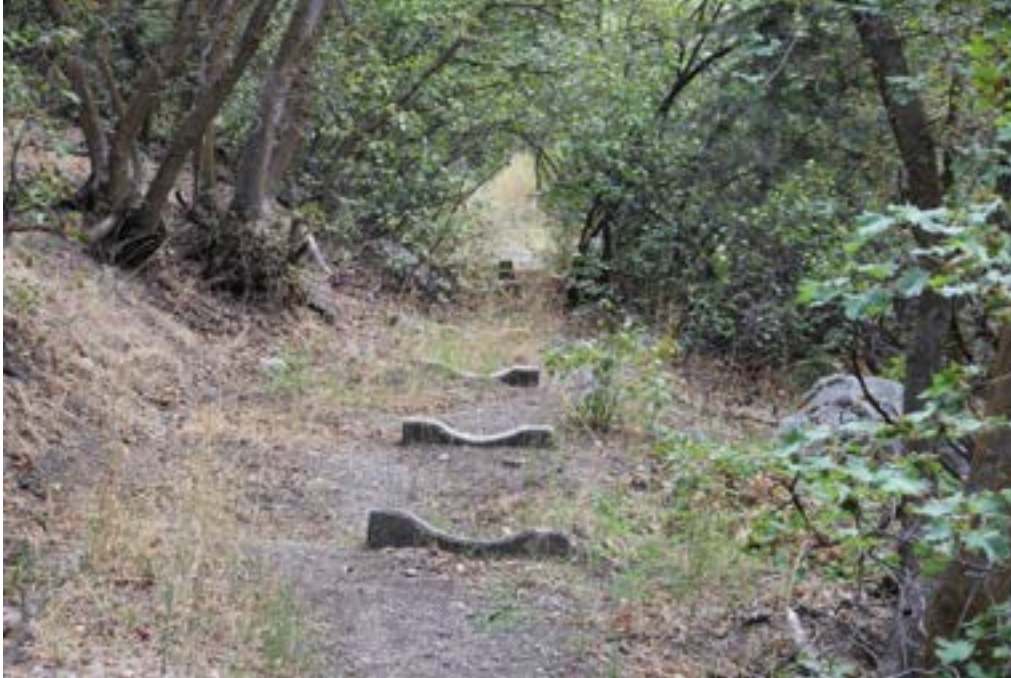
Photograph 7. Alpenbock Loop's Pipeline Trail section near Secret Garden showing concrete blocks formed to support a pipeline. Camera view east.
