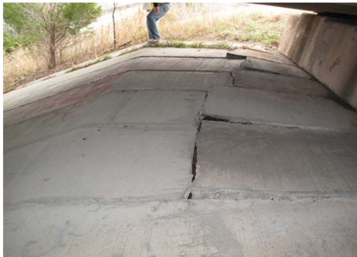
Figure 37. Cracks in the slope-wall
