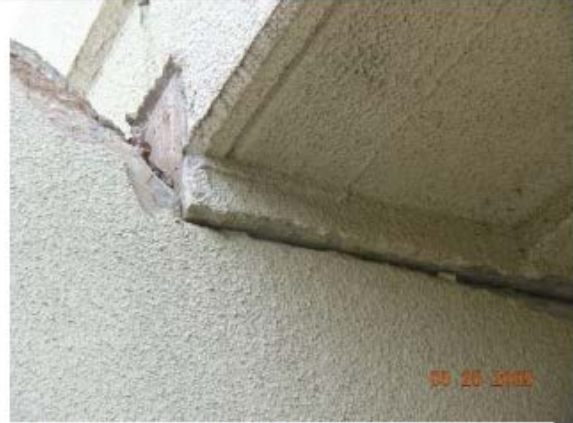
b) Approach slab overhang with eastern abutment wing wall spall
