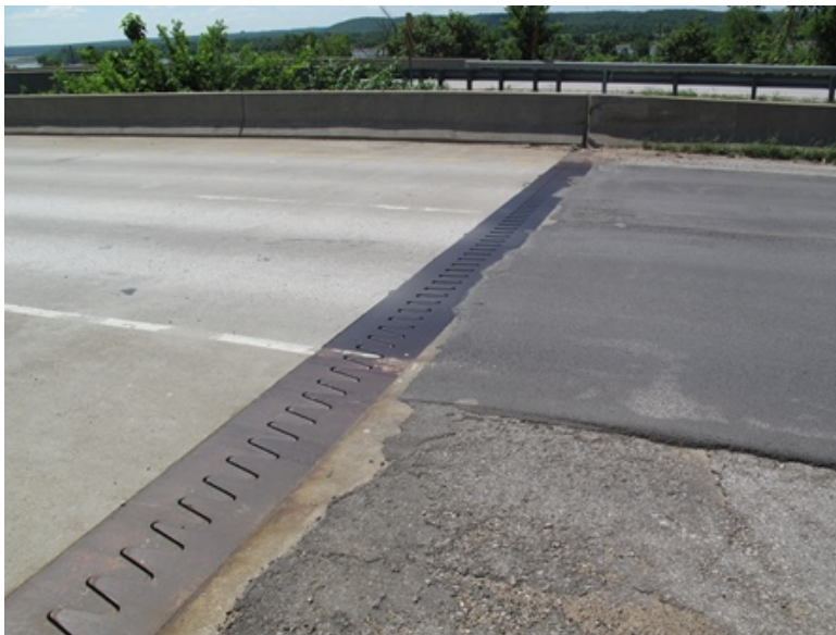
Figure 13. A closed expansion joint on the Shell Creek Bridge
