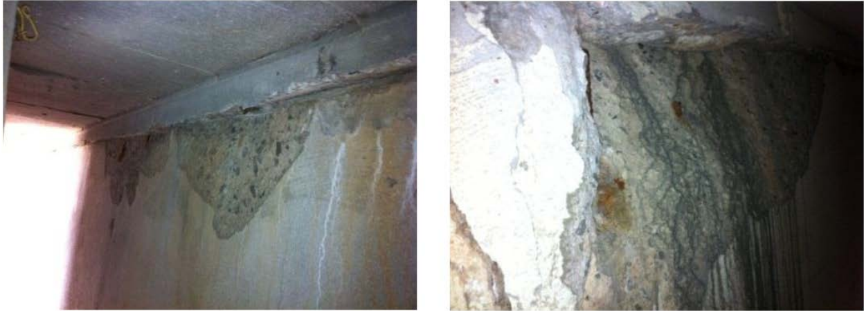
Figure 91. U-shaped cracking at 19 th Street/I-35 Bridge eastern abutment back wall in 2011
