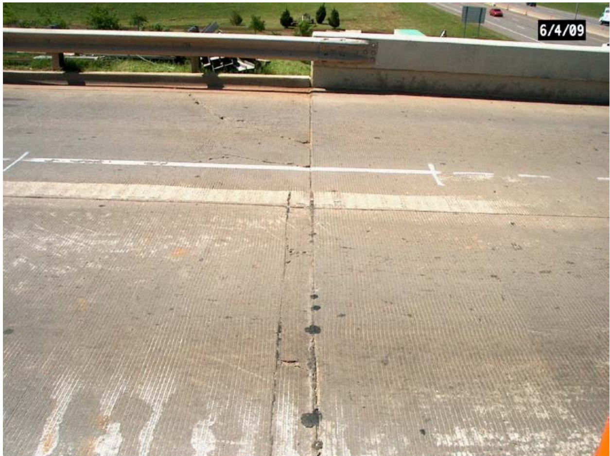
Figure 90. Cracking of the south eastern approach slab adjacent to south bridge deck in 2009
