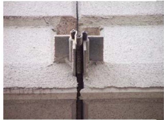
d) Center expansion joint on the South Bridge at 19 th Street (close up)
