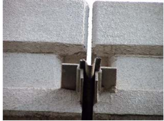
b) Center expansion joint on the North Bridge at 19 th Street (close up)
