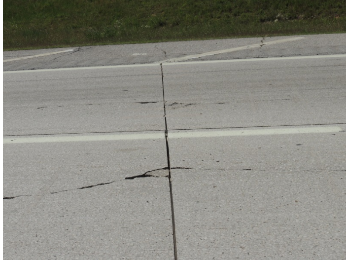
Figure 11. Picture of Longitudinal Cracking on I-40.
