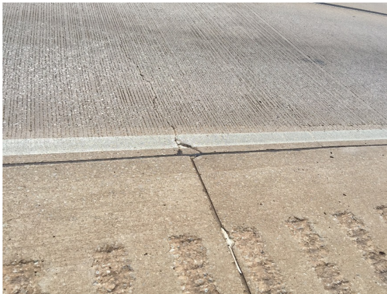
Figure 15. Picture of a Shoulder Joint Coincided with a Transverse Crack from I-35 SB.
