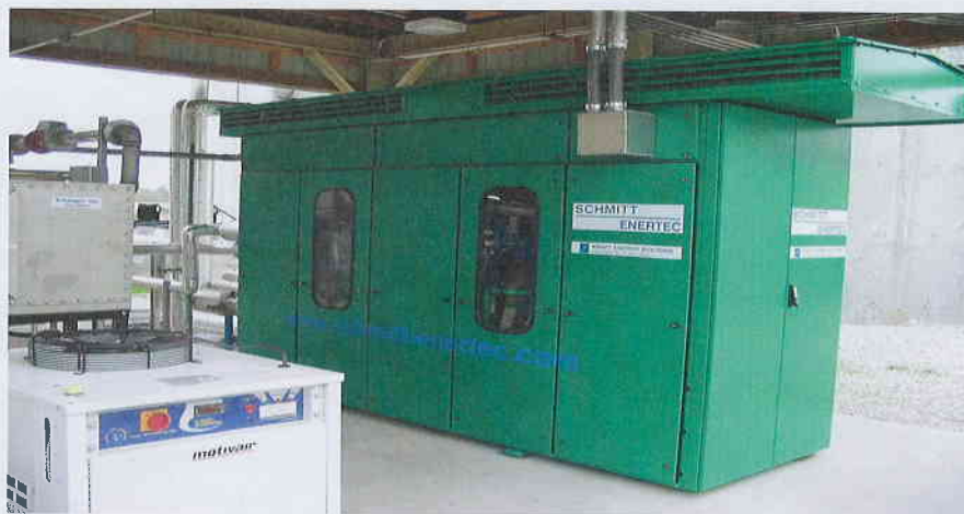
The Landis Sewerage Authority Wastewater Treatment Plant in Vineland, N.J., used a liquid booster to increase its methane production. The authority uses the methane to run this 185-kW Schmitt-Enertec (Mendig, Germany) generator as part of its combined heat and power system.
