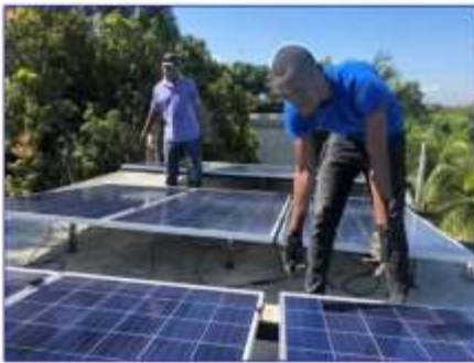
Salomon Asmath, LCS alumnus class of 1998 and partner at Energy Central (left) with Claseen, a technician with Energy Central, installing solar panels on the roof of the Radia Laboratory of Science and Technology.
